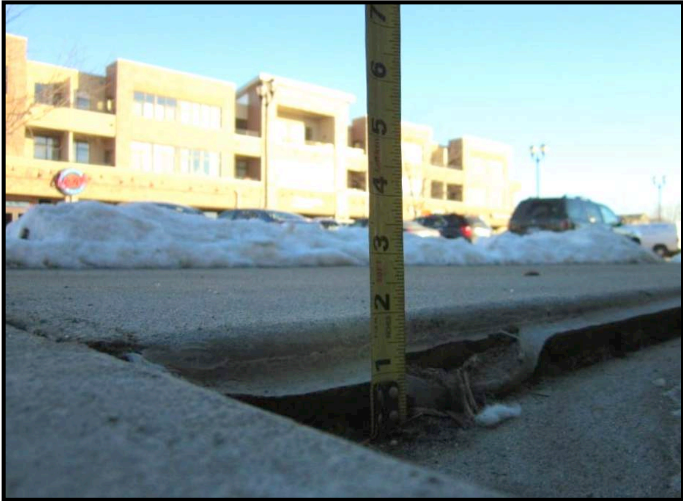
Slab settled 2", broken hand
