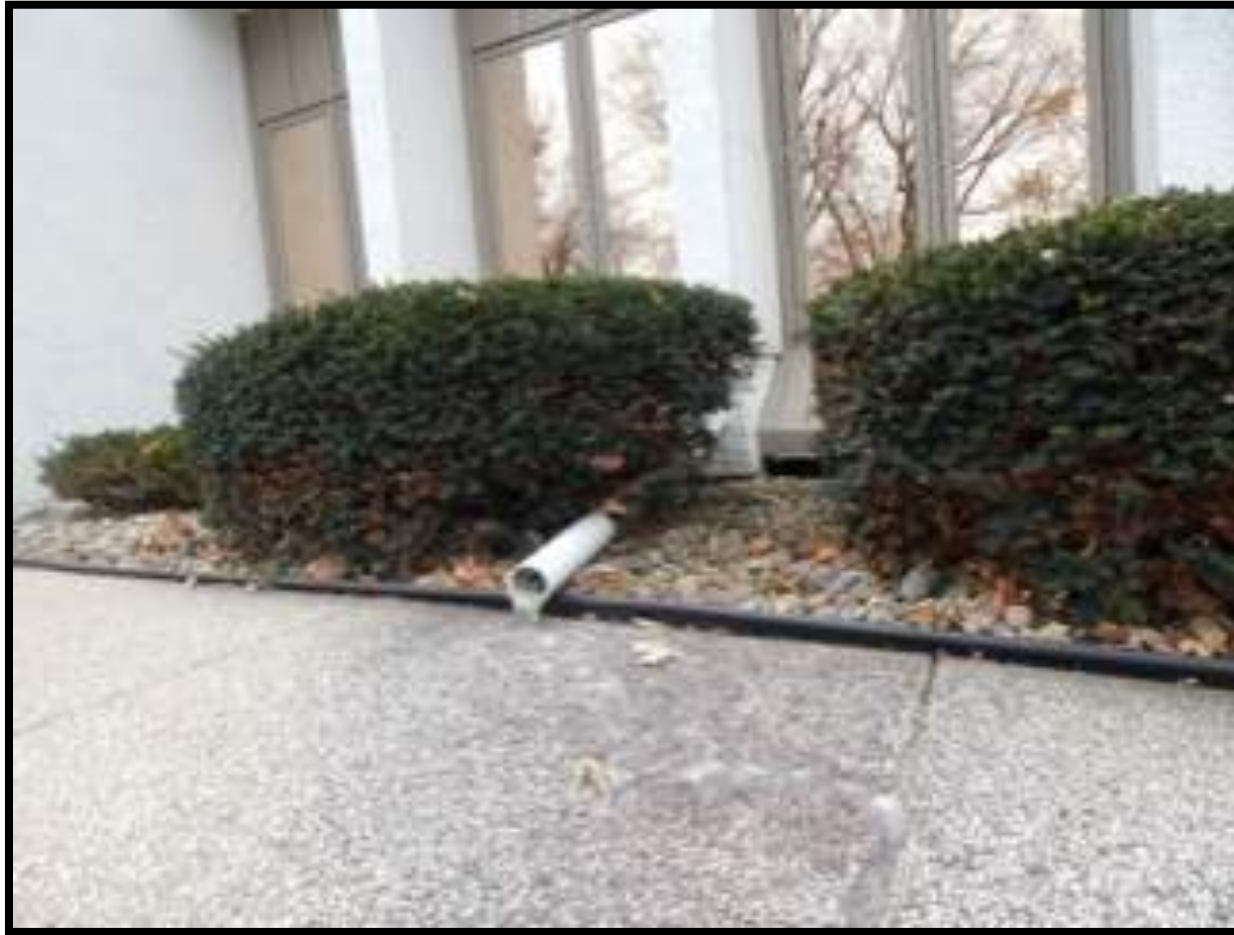
Brain Injury Facility - Poor drainage design
